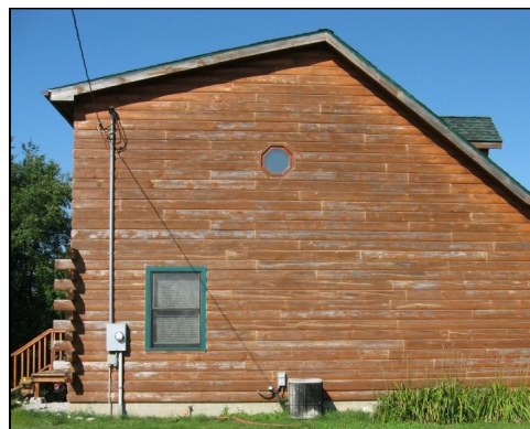
Example of Mold & Mildew
