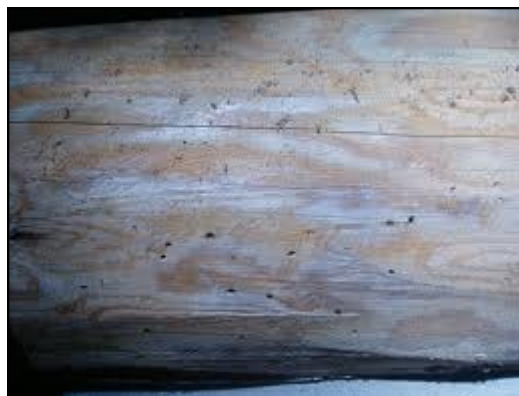
Evidence of Wood Destroying Insects
